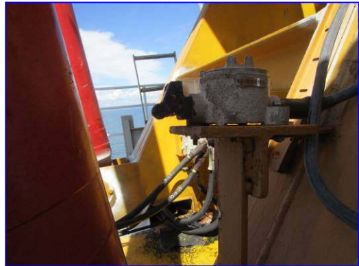
Boom Limit Switch
