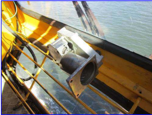
Cabin Glass Wiper not function, Wiper motor was broken shall be repaired
