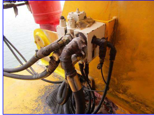
Luff Control Valve for Boom Cylinder Found Leaking
